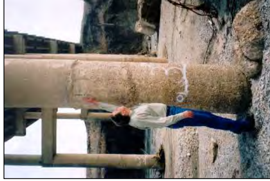
SH 34 BRIDGE (NOTE THE EROSION SINCE BRIDGE CONSTRUCTED IN 1960)
