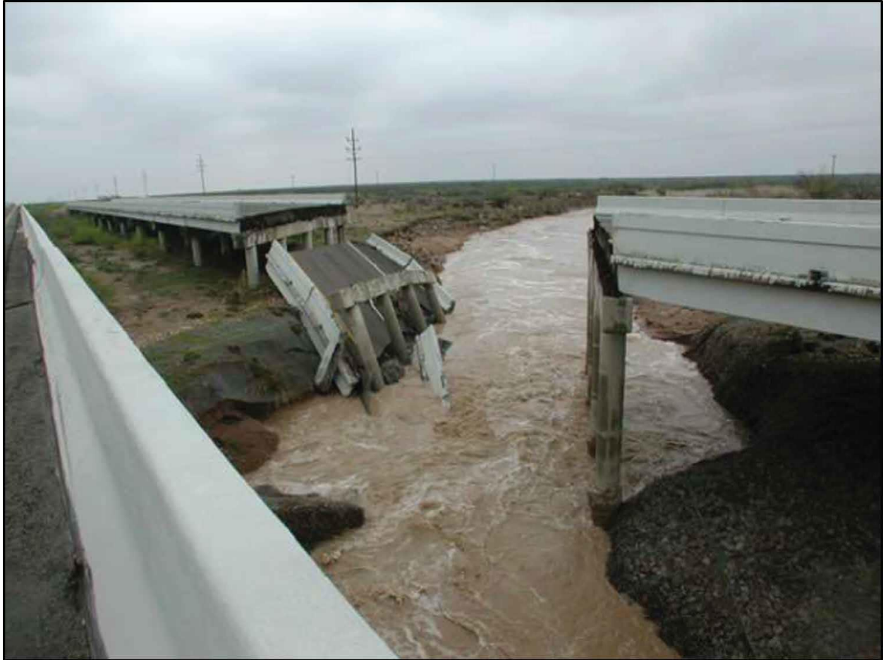
April 2004 flood caused this I-20 bridge over Salt Draw to collapse, located between Toyah and Pecos. Source: NOAA and NWS; https://www.weather.gov/maf/2004_04_02_SevereWeather
