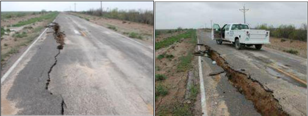
Sinkholes formed along this County Road southwest of Pecos, Texas during the April 2004 storm event. Source: NOAA and NWS; https://www.weather.gov/maf/2004_04_02_SevereWeather
