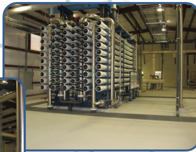
Reverse Osmosis Trains
