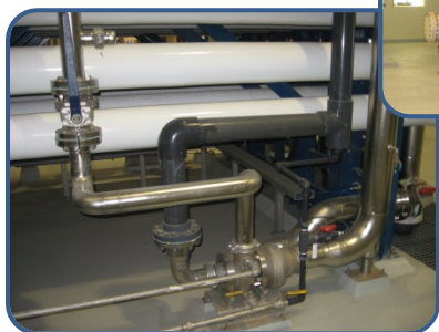
Energy Recovery Device
