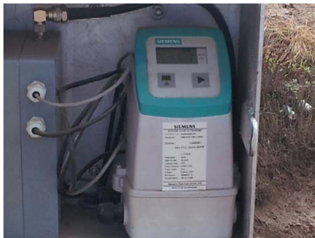
Telemetry Unit (left) and Flow Meter (right) Inside Vandal Box
