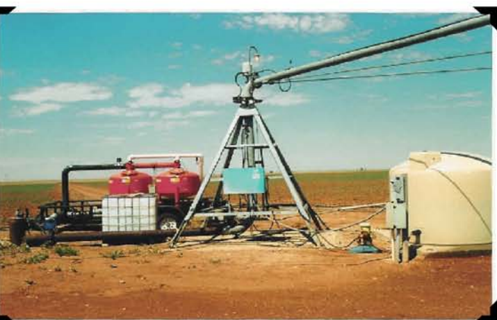
The filter system (left) and a tank beside the center pivot system.
