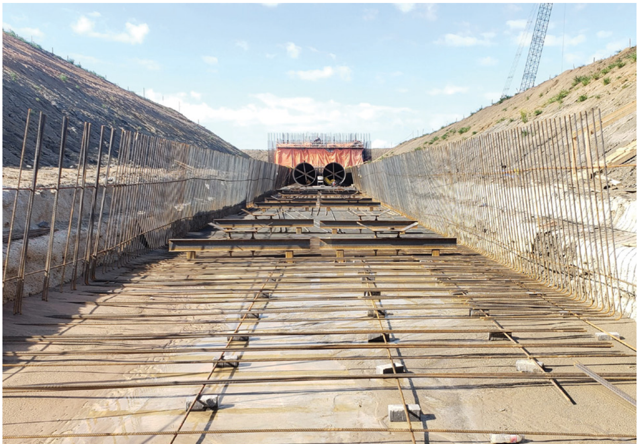
Intake structure at Bois d'Arc Lake; photo courtesy of North Texas Municipal Water District
